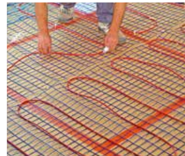
Heating cables connection.
